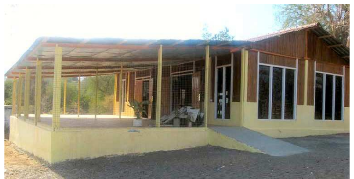
The Atabae Community Health Centre building is now complete and considered the best constructed building in Atabae.
